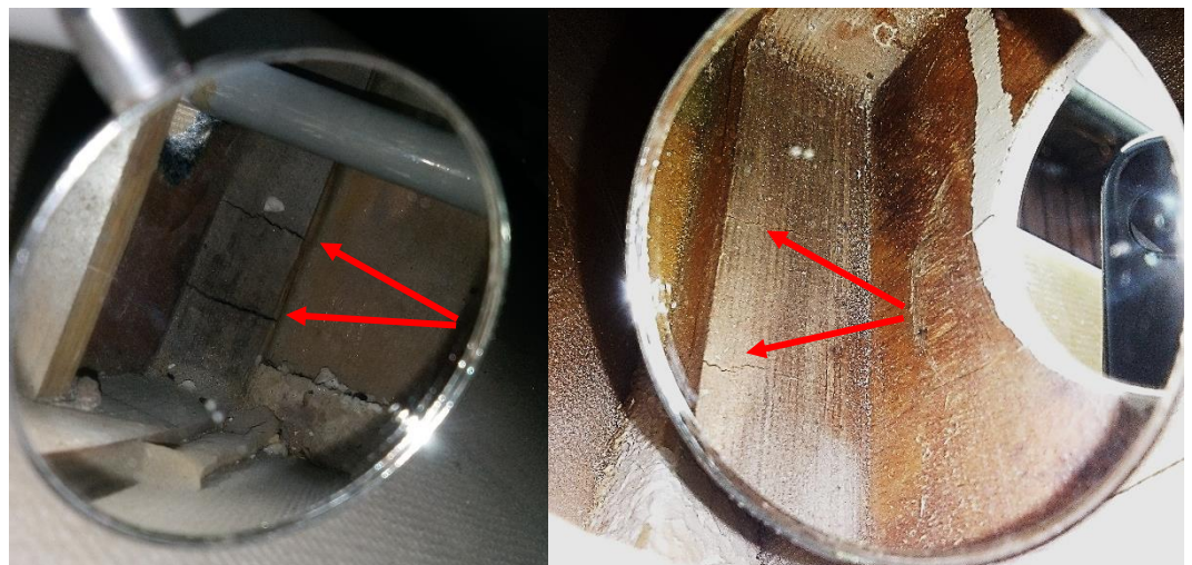
Fig. 1: Cracks perpendicular to the root rib plane. Left: significant cracks, right: incipient cracks
