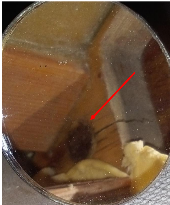
Fig. 6: Loose lift pin bushings
