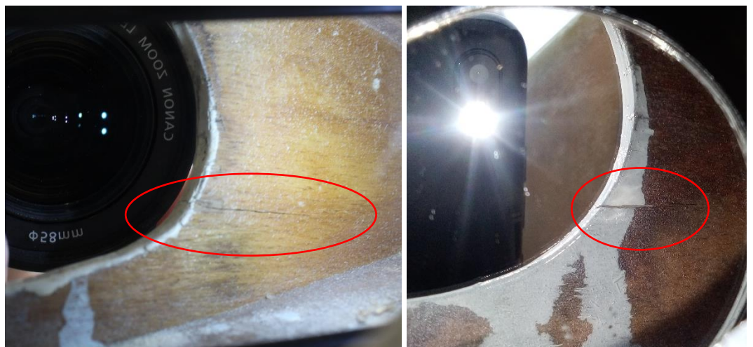
Fig. 4: Cracks in the shear wall
